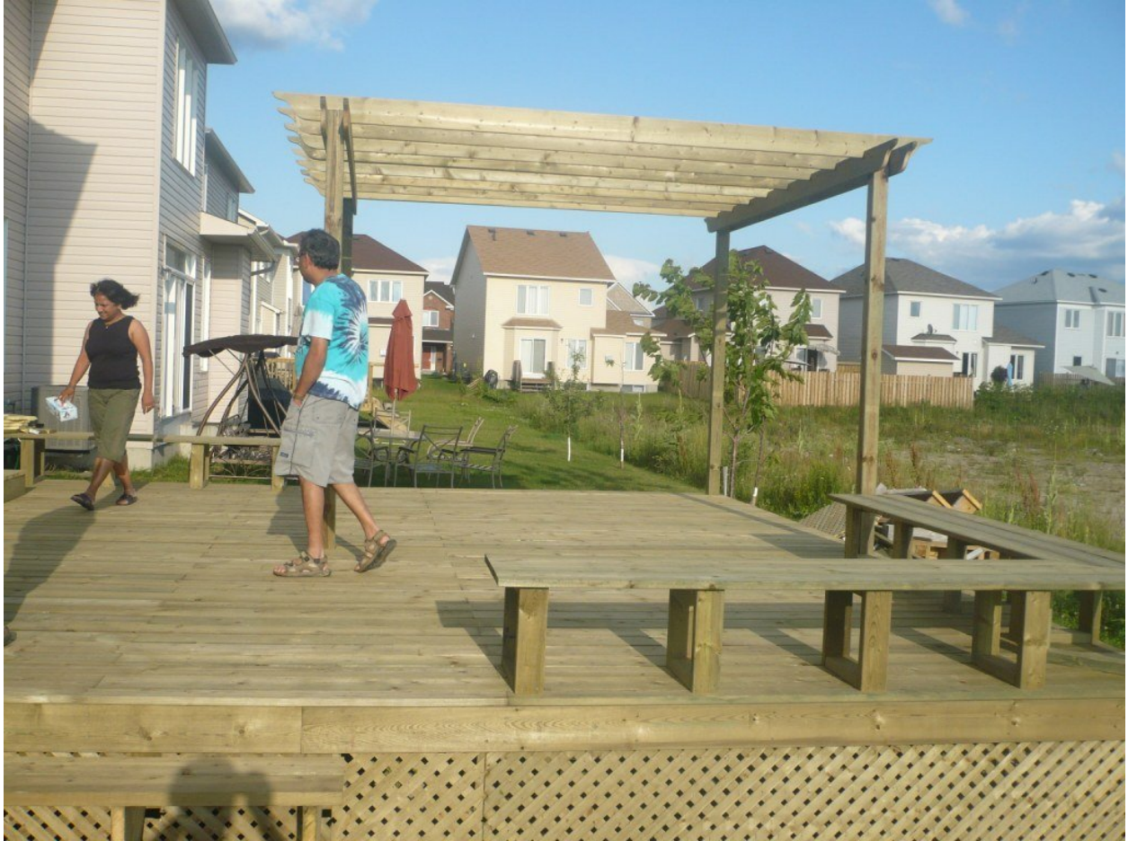
Figure 2: The first deck I built. When I first started I knew nothing about how to build a deck. I did 15 estimates until I finally booked this one. The cost to customer was $4500. I grossed $2500 profit from the job. When the job was presented to a competitor they told me I under bid. They would have charged $8000 for the deck and had a grossed 75% profit. The deck and fence business can be very lucrative.
